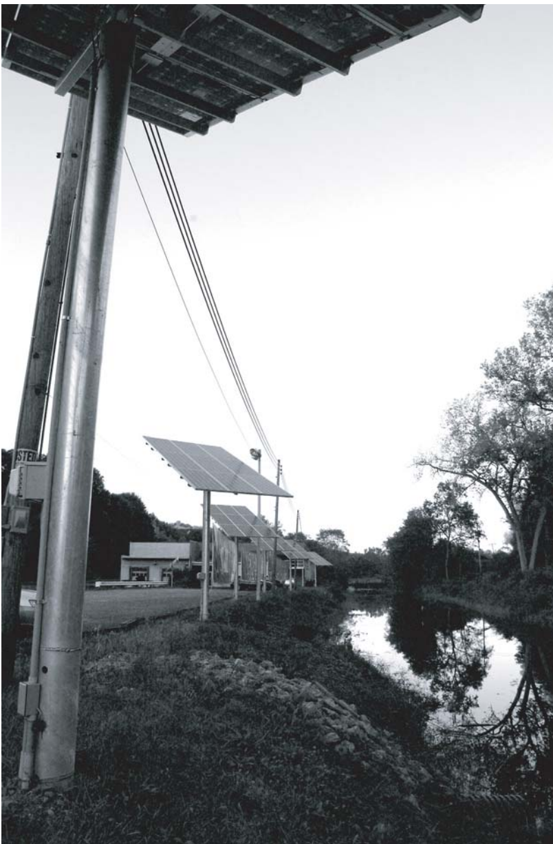
(ABOVE LEFT) SOLAR PANELS ON THE KLING MAGNETICS /SUNDOG SOLAR/SOLAQUA CAMPUS;
